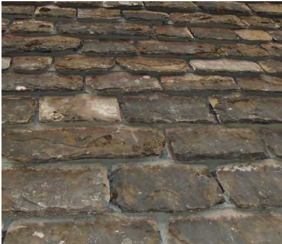
Laying of Horsham Stone slate roof with shadow slates and inconspicuous mortar
